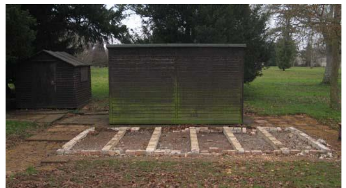
The supporting beams, seeing the light of day after forty years or so.
